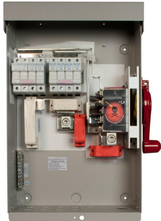
MNPV8HVMCM300 Kit fully installed.
