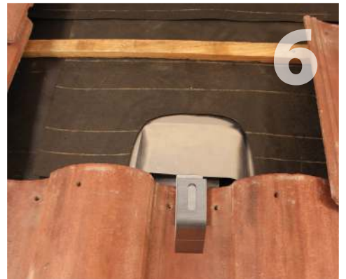
6 Waterproof at underlayment level according to roofing manufacturer instructions and Tile Roofing Institute Guidelines.
