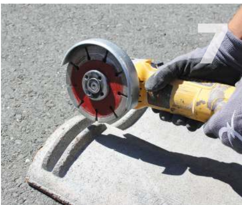
7 Cut a clearance notch in the weather guard lug using a grinder with a tuck point blade. Make sure the tile seats back down in its original position. Leave at least 1/4" of tile to prevent breaking through.
