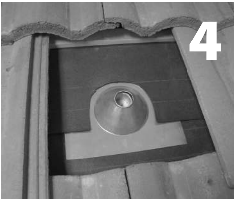
Install subflashing. Waterproof at underlayment level according to roofing manufacturer instructions and Tile Roofing Institute Guidelines.
