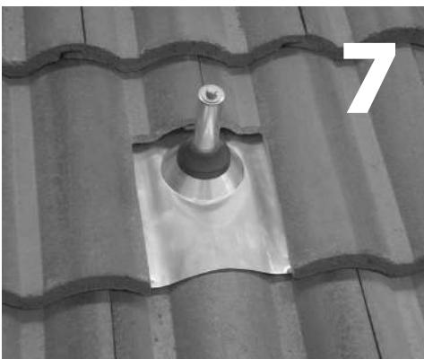
Another acceptable method is to notch the tile and install the 18"x18" flashing under the tiles. This is very common in standard roofing.
