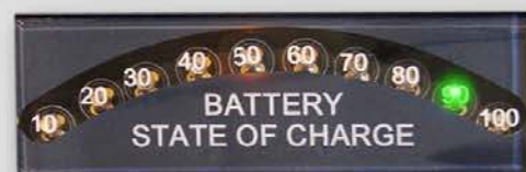
Batteries have a 90% charge
