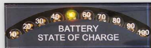
Batteries have a 50% charge
